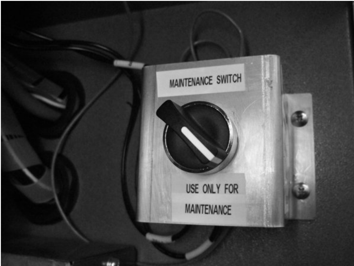
Figure 6.2: Chute Maintenance Switch
